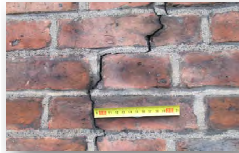
Cracking in No. 28
