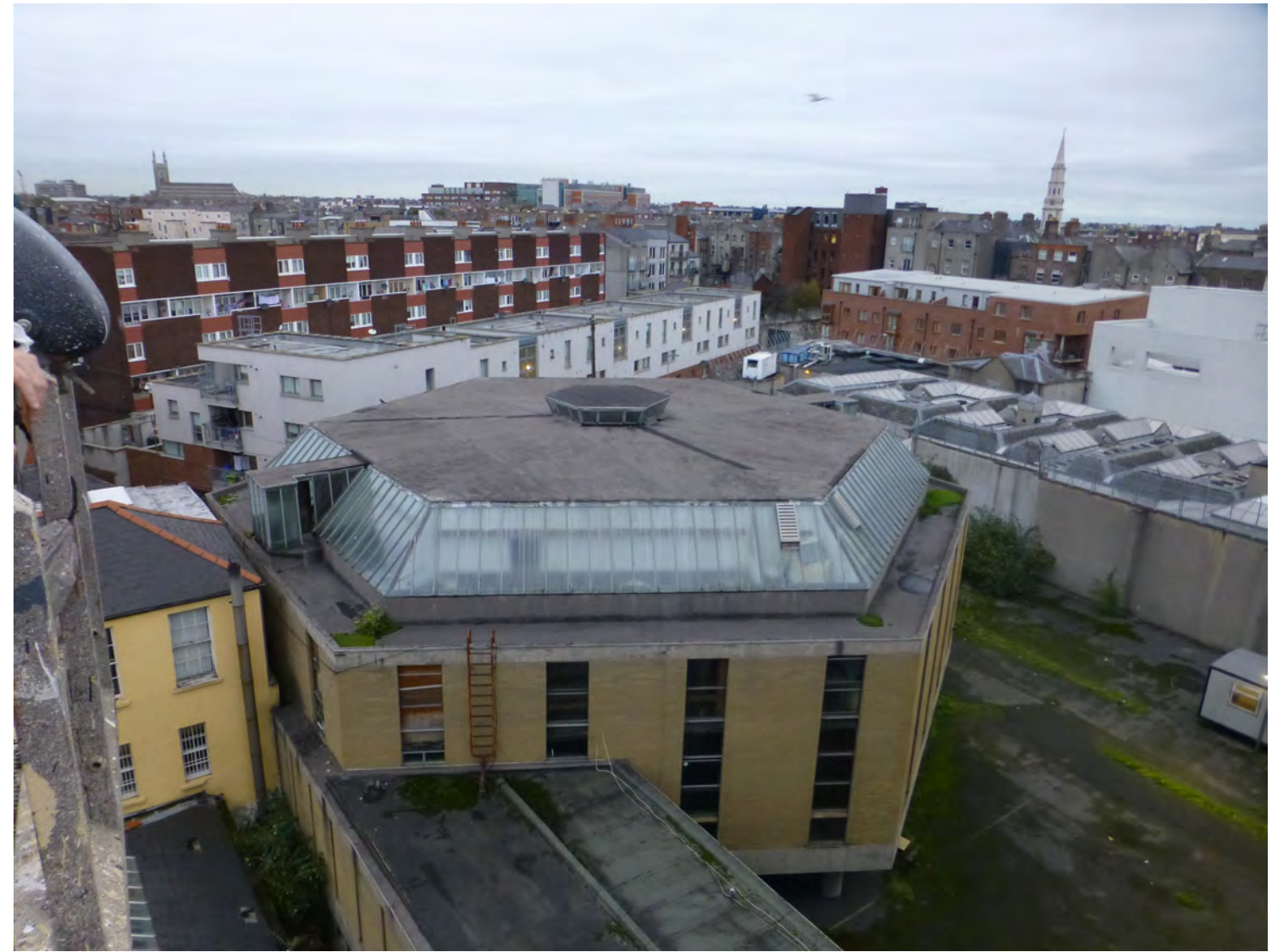
Fig 7.24: View from hoist/roof of No 28 towards the 1960's octagonal Amharclan building with its partially glazed set-back roof. To the right is the roof of the 1930's Hugh Lane Gallery extension and in the background, the Sheridan Court housing scheme.
