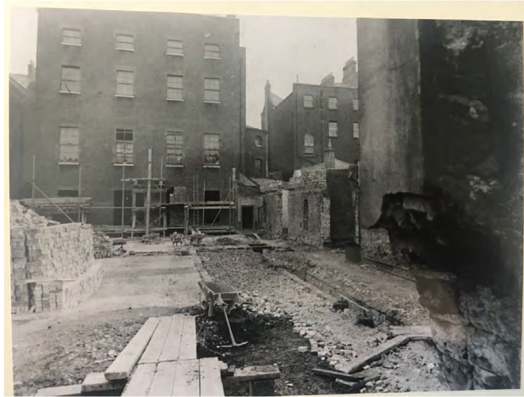
Fig.2.41 Photograph, c. 1929 of the rear of Charlemont House following demolition of structures to facilitate construction of the Municipal Gallery (source Irish Architectural Archive).
