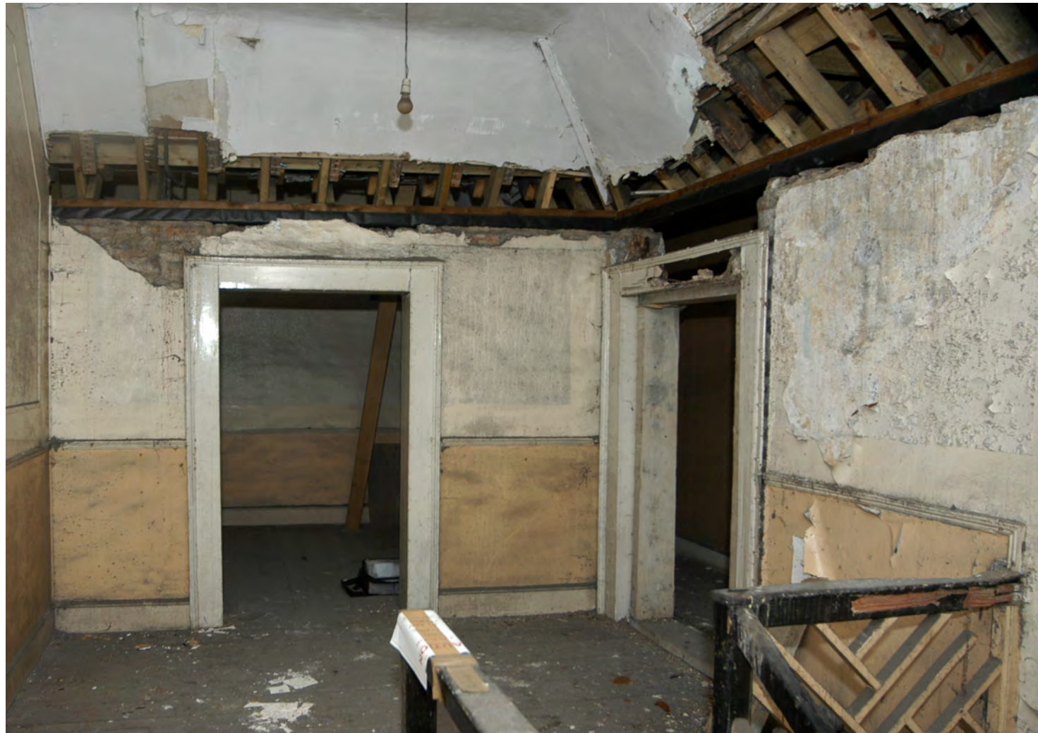
Fig 3.5: No 23 third floor showing typical areas of decay - temporary repairs carried out to exposed rafter ends)
