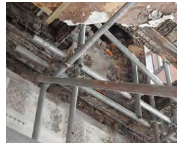
Figs 3.2; 3.3; 3.4: above: No 28 damagee caused by water ingress and where fireplace hearth has fallen through damaging staircase below.
